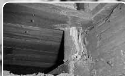
Drywood termites attack dry, undecayed wood.
