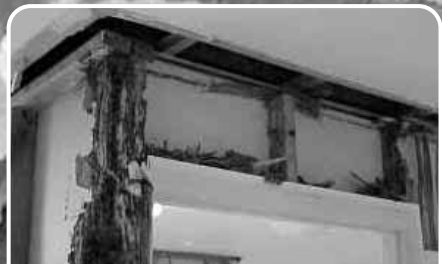
Subterranean termites consume the wood from the inside out
