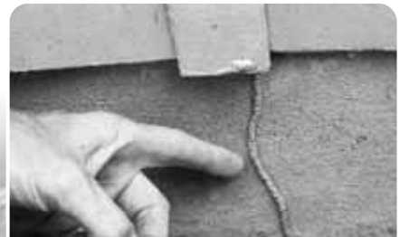
Mud trails shelter subterranean termites on the move
